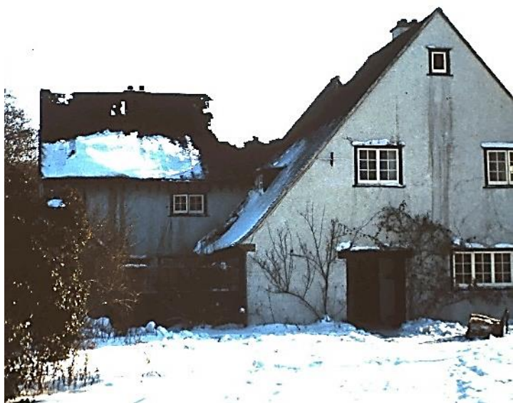
Monks Barn after the fire
